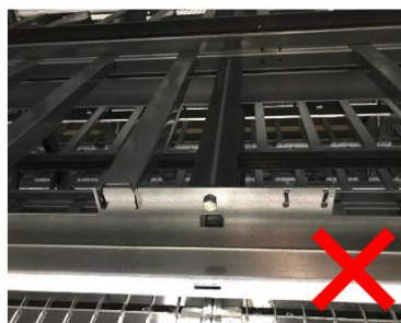
Support profile on the right missing
